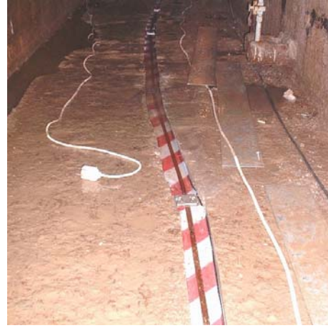
Figure 8: SMARTape installation in the inspection gallery.
